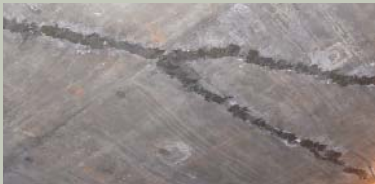
◀ Visible crack in concrete.
